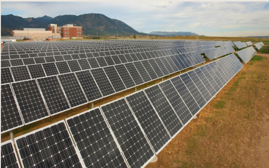
Battalion Headquarters solar array at Fort Carson, CO (photo: Harry Weddington, USACE).
